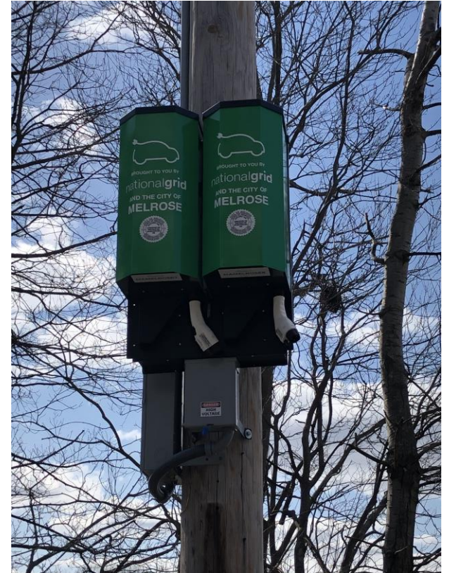
Dual pole-mounted charging station installed in Melrose, MA
